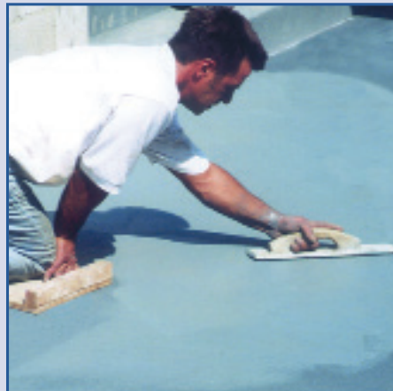
1. Finish concrete following normal practices, using Bon True Color™ Hardener or Ironox™ Integral Color.
